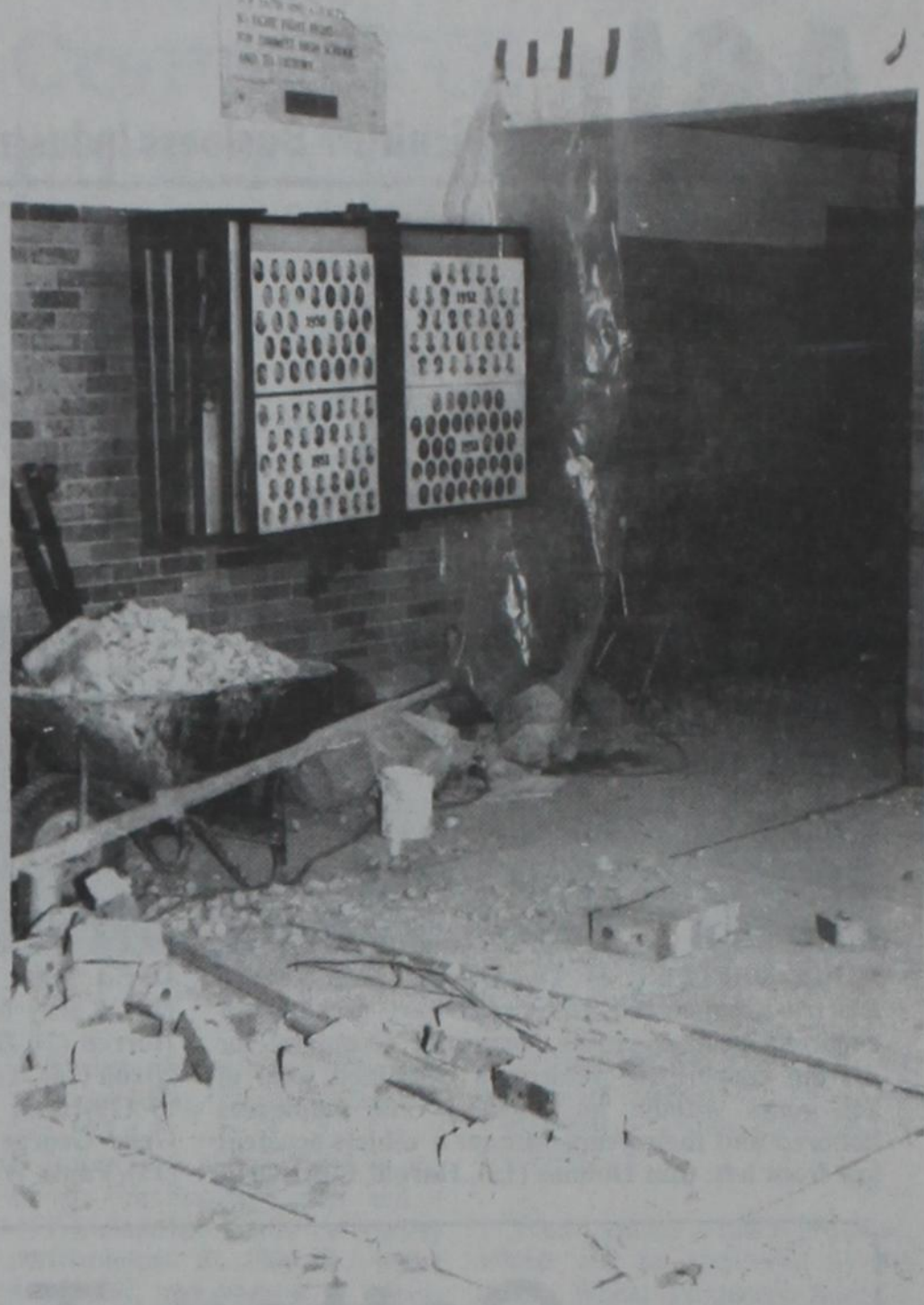
ALMOST FINISHED —Although some bricks and mortar remain in the high school's foyer, Assistant Principal Lyman Schroeder said the remaining construction won't affect classes, which begin Aug. 26. All exterior work is completed, and the construction crews are now detailing the interior, he said. Schroeder said every teacher should have a classroom by the first class day.
