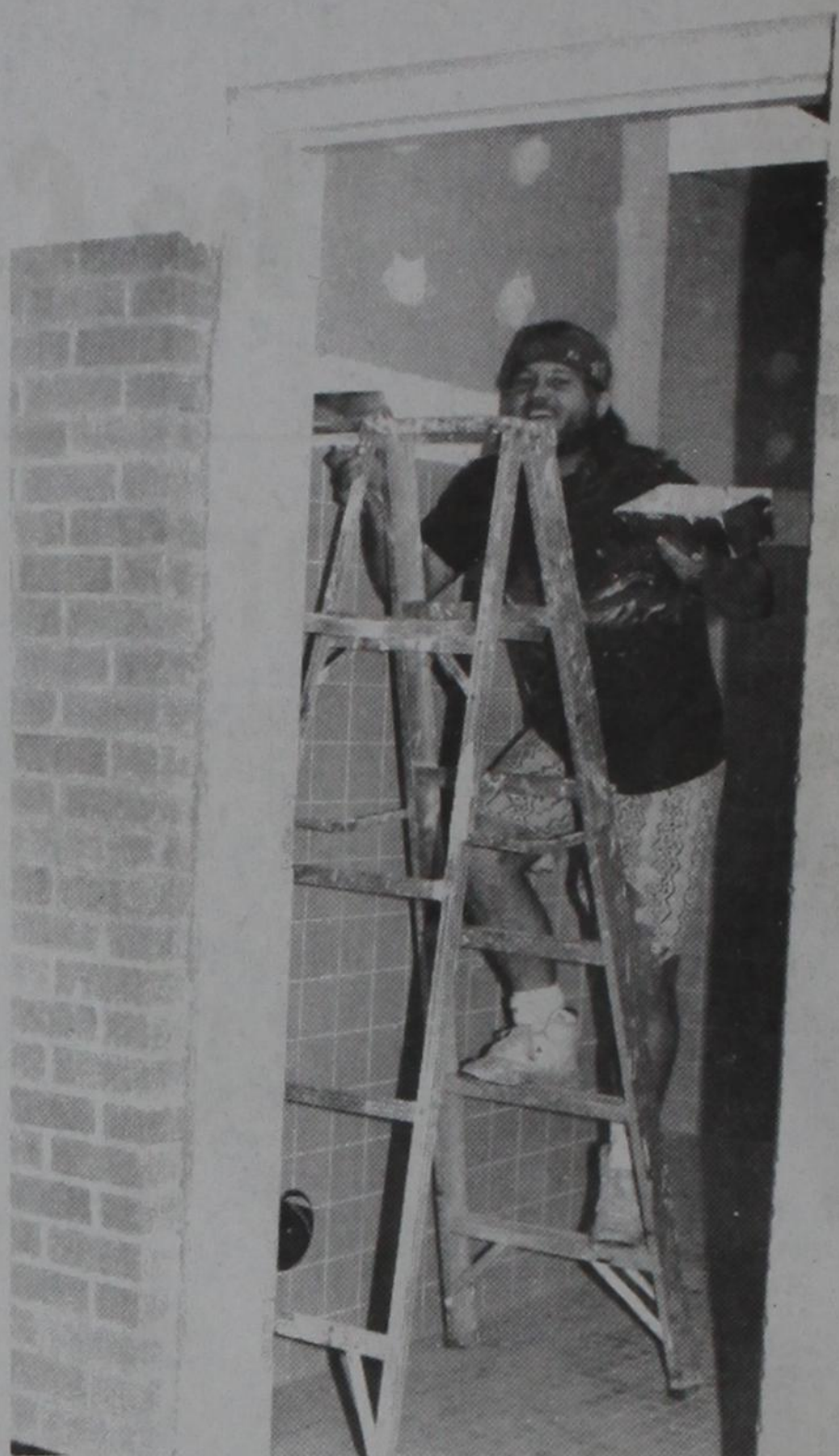
AND THE WORK GOES ON—Mike Northcott of S&R Contractors of Lubbock is plastering restroom walls in the new classroom addition on the south side of the Dimmitt High School. The classrooms are currently in use, but the library, restrooms and finish work in the halls are still incomplete. DHS Principal R.L. Stockstill said the work should be completed within a week or so if everything goes according to plan.
