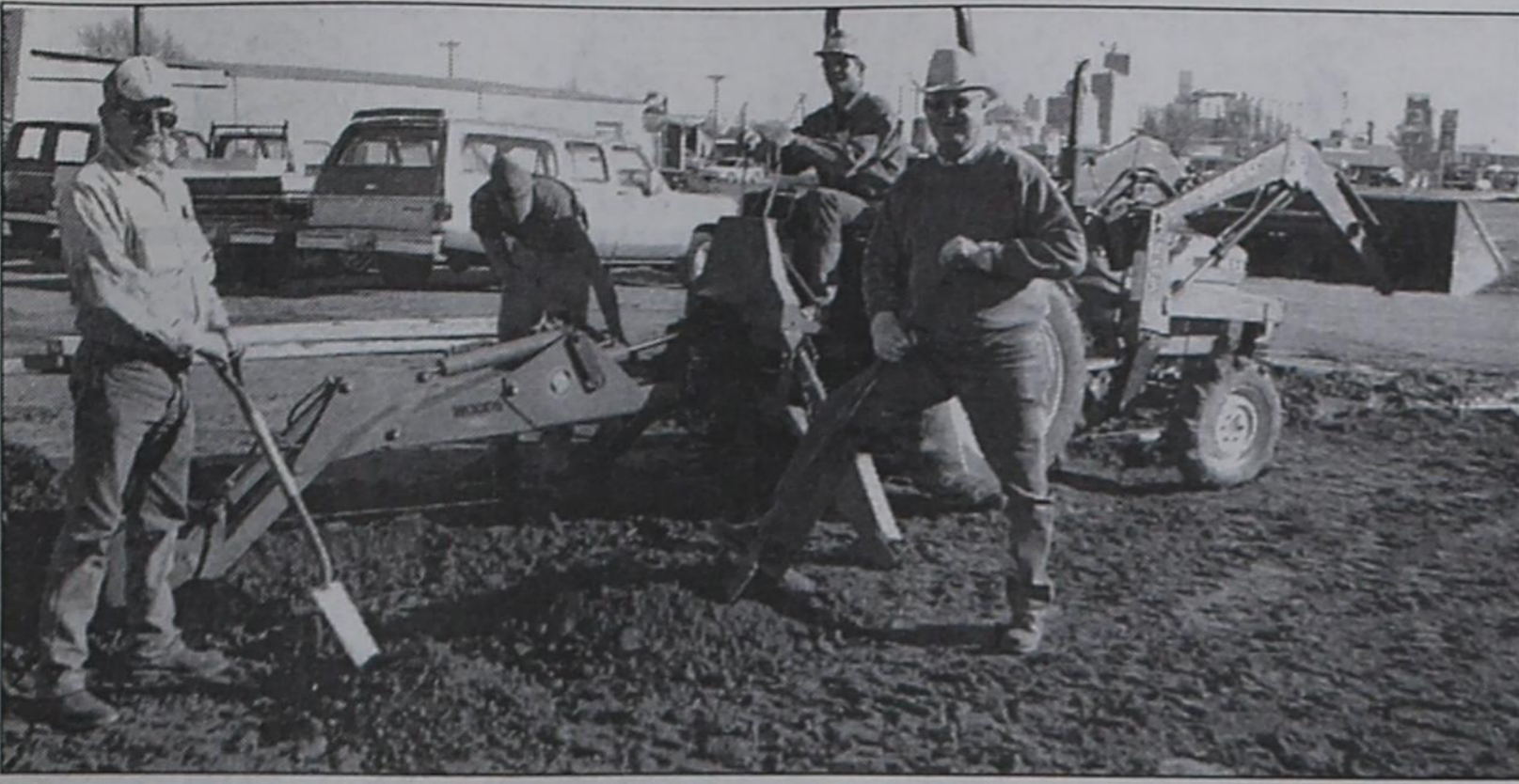
DIMMITT LAUNDRY GROUNDBREAKING —In about 45 days, partners Donny McDaniel (left) and Avery Thrasher (right) expect to open a laundromat in north Dimmitt just behind Thrasher Auto Sales. The 40 x 50-foot building eventually will house 30 washers and 10 dryers, as well as various vending
