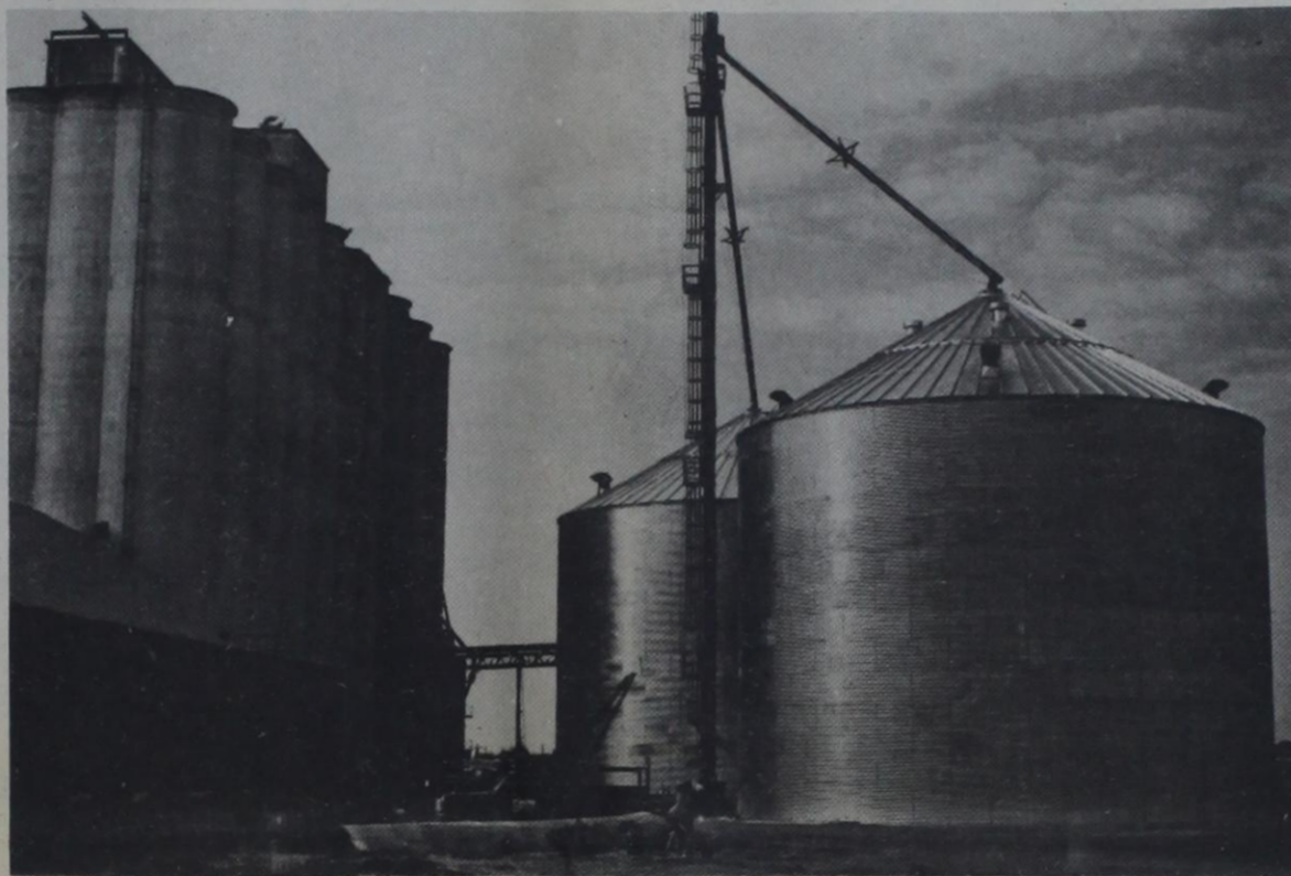
NEW STEEL STORAGE TANKS GOING UP AT BRUEGEL & SONS, DIMMITT . . . Will be ready in time for corn and milo harvest
