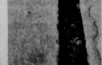
DIVIDED STREET—A huge crack runs along a street in Puerto Montt, Chile, hit hard by earthquakes.
