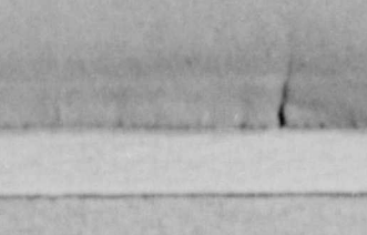
DIVIDED STREET—A huge crack runs along a street in Puerto Montt, Chile, hit hard by earthquakes.
