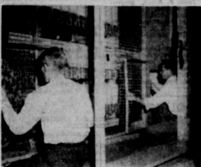
FROM MANUAL TO DIA - Thurman Rucker of Fort Worth, left, and Aaron Howton of Ranger, pull the blocking tools from line relays...
