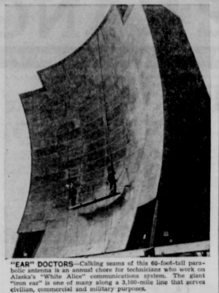
"EAR" DOCTORS—Calking seams of this 60-foot-tall parabolic antenna is an annual chore for technicians who work on Alaska "White Alice" communications system. The giant "iron ear" is one of many along a 3,100-mile line that serves civilian, commercial and military purposes.
