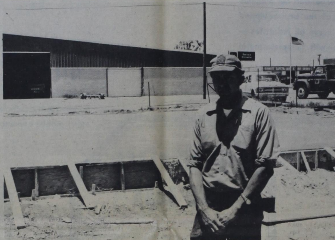
Jim Cleavinger, president and service manager of C&S Equipment Co., shows the site of a new 40 x 50 ft. steel building which will go up soon to provide more space for set-up and repair of John Deere equipment. The new building will be just east of the plant's main building, and will be furnished with specialized equipment for servicing John Deere farm machines.
