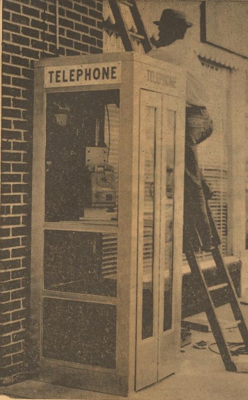
NEW PAY TELEPHONE booth installed last week between Thomas Jewelry and City Drug by West Texas Telephone Company now offers pay telephone facilities for downtown shoppers. —Cowan staff photo
