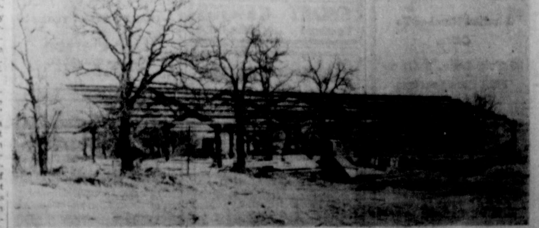
CLUBHOUSE IS GOING UP—Folks driving around Lake Leon in the last few days have been surprised at the progress made on the new Lake Cedar Country Clubhouse during the past week.
