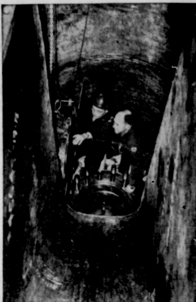
ATOMIC HEART — Master Sergeant Charles R. Feayear (right) of Saginaw, Mich., stands over the tank that will hold the nuclear material in the package power reactor plant at Fort Belvoir, Va. Specialist Third Class Hendrick T. Rosenbrock of Hoboken, N.J., engineer draftee, is his guide. Feayear has been university-trained by the Army to qualify as a plant superintendent.
