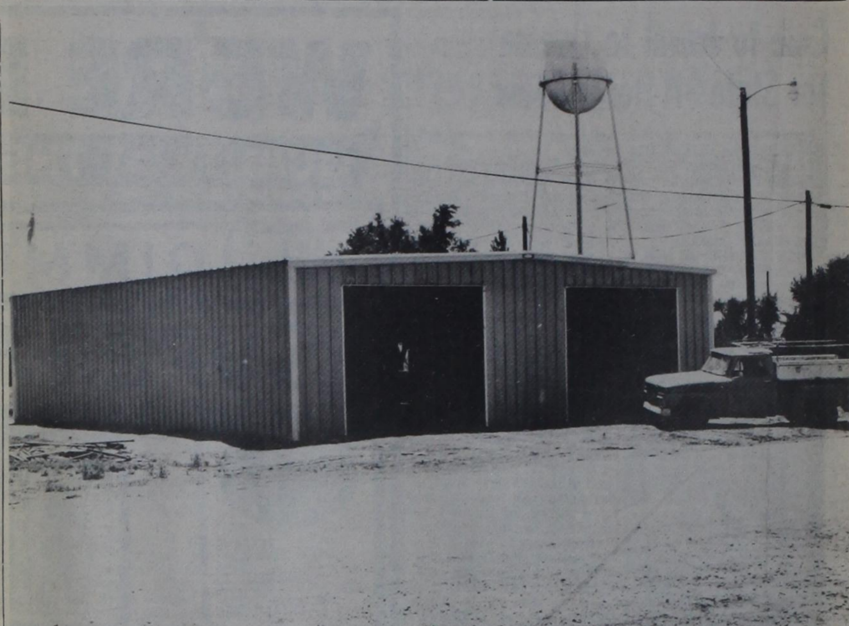
AWAITING DOORS—Nazareth's new fire station has gone up quickly and is now awaiting doors for the front. The construction was financed by several townspeople who signed notes on the building, and the actual construction has been performed by citizens of the young city.
