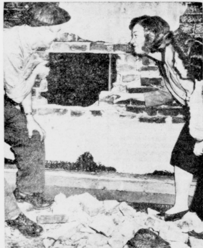
HOLE IN THE WALL —These three Philadelphians examine the damage done by thieves who chiseled through this 18-inch wall of a Philadelphia grocery company. The burglars escaped with $1800 cash and the company's books.
