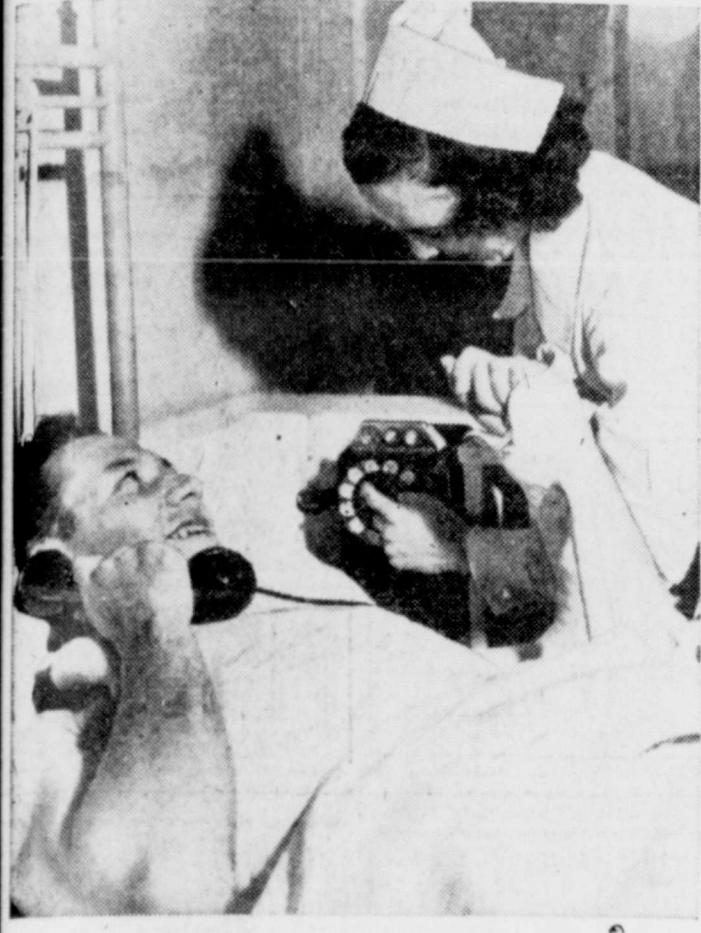
ONE PHONE, COMING UP—Home is no further than bedside, thanks to "Telecars," installed in Veterans Hospital at San Francisco. Portable telephone is plugged into wall outlet near bed of Harry Karulow and nurse dials his number.
