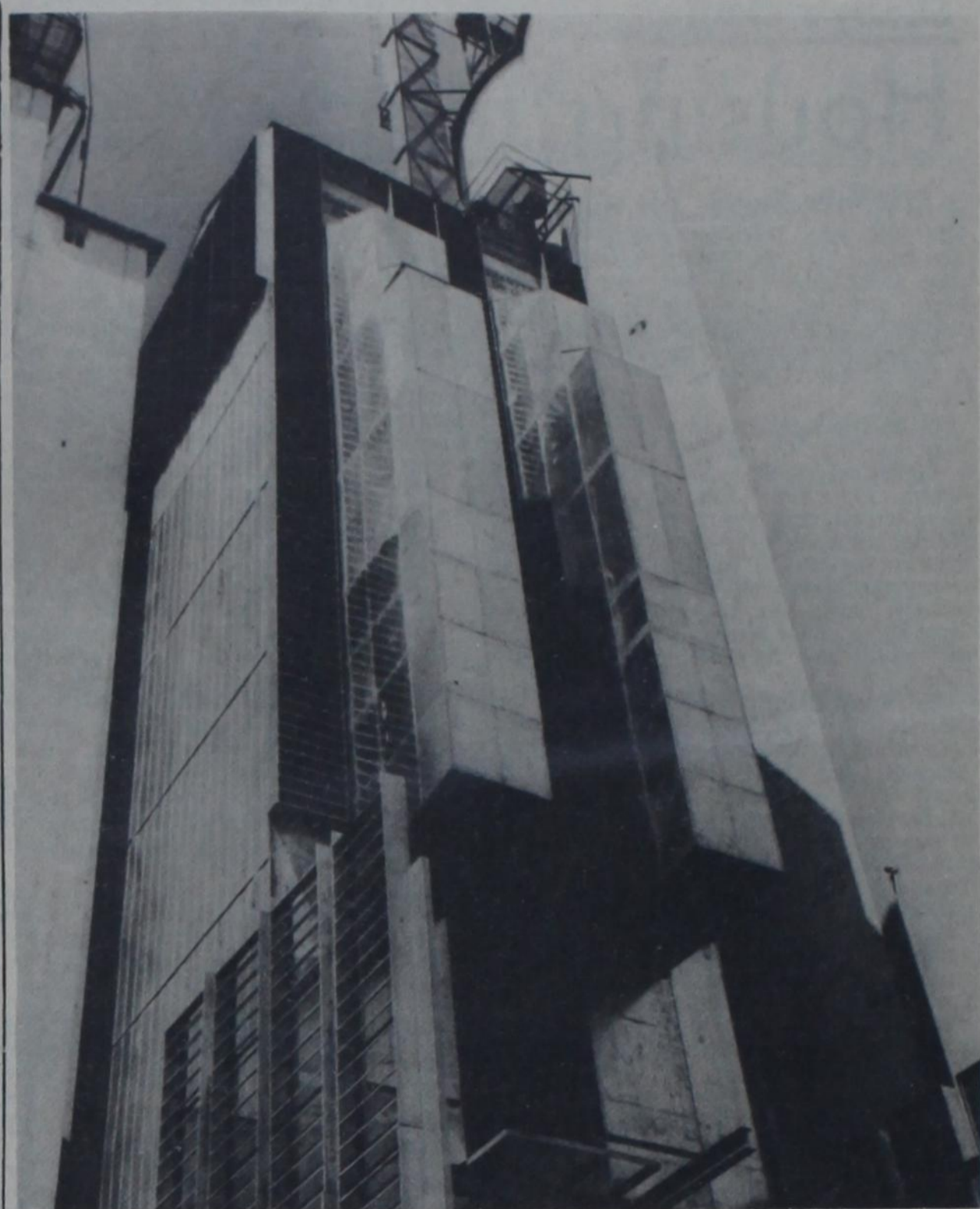
THE NATION'S BIGGEST CORN DRYER is in the final stages of installation at Dimmitt Agri Industries, Inc., and is expected to go into operation next week. Manufactured by Carter-Day Manufacturing Co., the Shanzer type dryer is the biggest model built. It dries 6,000 bushels per hour, removing five points from the corn's moisture content, and will enable DAI to handle a limited amount of corn with up to 25 per-
