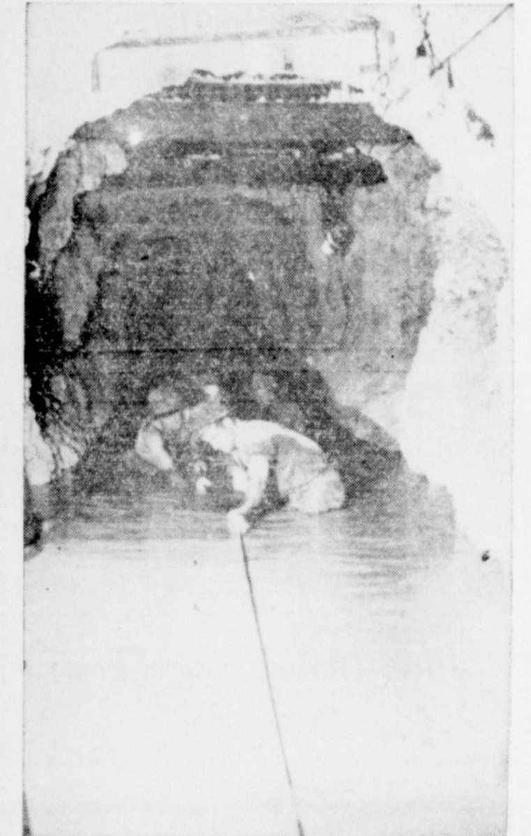
WATER FOR FLEET —Told by geologists that heretofore untapped source of water lay underground on Guam, Seabees of 5th Naval Construction Brigade built tunnel to reach millions of gallons needed by fleet. Here they're working on tunnel.
