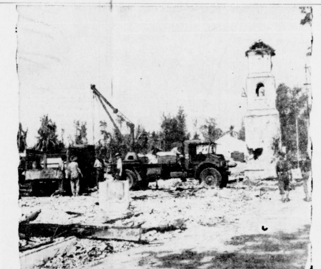
IMMEDIATE RECONSTRUCTION —Even before fighting on island is over, Aussie engineers build Victoria, main settlement on Labuan, Borneo. Town was practically destroyed by U. Navy gunfire which preceded landings. Here Bulldozers clear rubble from streets
