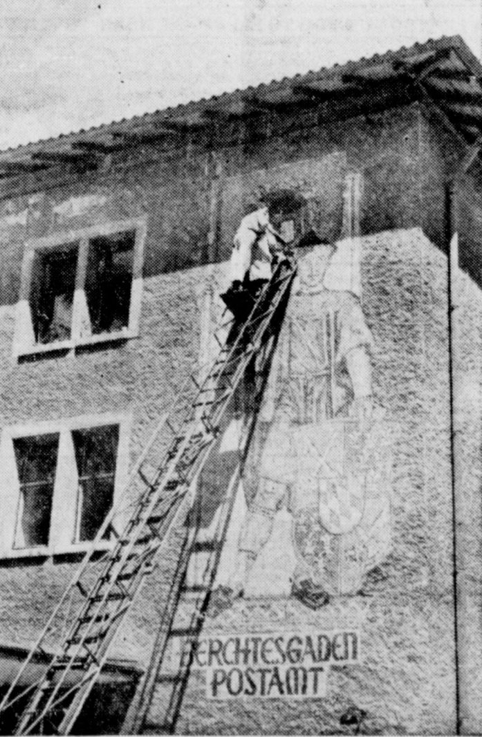
DOWN WITH THE OLD—Removing all the swastikas in occupied Germany is no small job, but Allies are systematically replacing Nazi symbols with those of peace. Here a painter blacks out insignia of the Third Reich that was emblazoned on side of Berchtesgaden post office.
