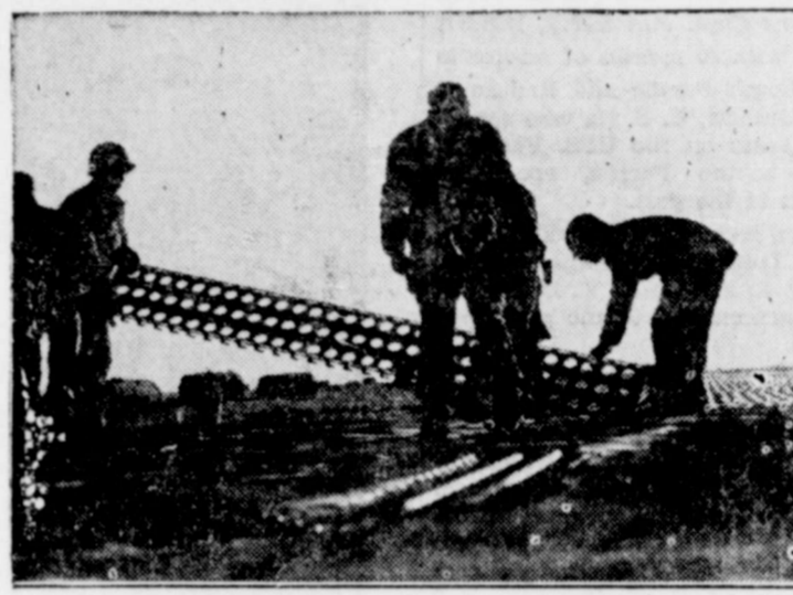
Released by U. S. War Department, Bureau of Public Relations. AVIATION ENGINEERS WORK IN THE DAWN—Silhouetted against the morning sky members of this Ninth Air Force Engineer Aviation Battalion fasten the final sections of steel planking in completing runway on German soil.
