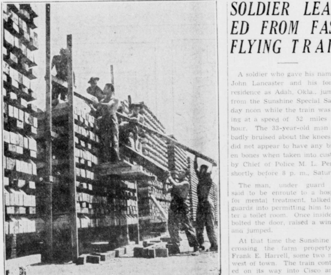
HIGHER AND HIGHER—These Italian Service Unit men at the port of embarkation, Charleston, S. C., are stacking millions of board feet of lumber which has been reclaimed from scrap. At this port alone it is estimated that $75,000 worth of lumber has been reclaimed.
