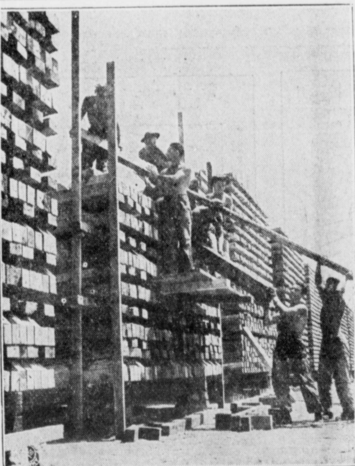
Released by U. S. War Department, Bureau of Public Relations HIGHER AND HIGHER —These Italian Service Unit men at the port of embarkation, Charleston, S. C., are stacking millions of board feet of lumber which has been reclaimed from scrap. At this port alone it is estimated that $75,000 worth of lumber has been reclaimed.
