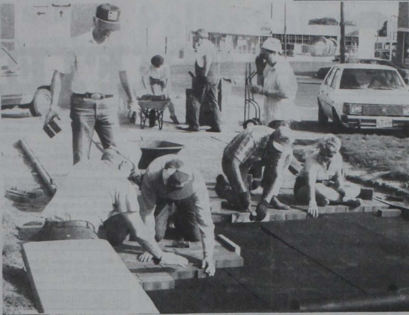
FOLLOW THE RED BRICK WALKWAY —A crew of about 20 showed up Saturday to help lay the bricks for the plaza area surrounding the Centennial Gazebo on the northwest corner of the courthouse square in Dimmitt. Working here are (standing, from left) Percy Parsons, Wanda Stevens, Bill Sava, centennial co-chairman, and Darlene Collins; and
