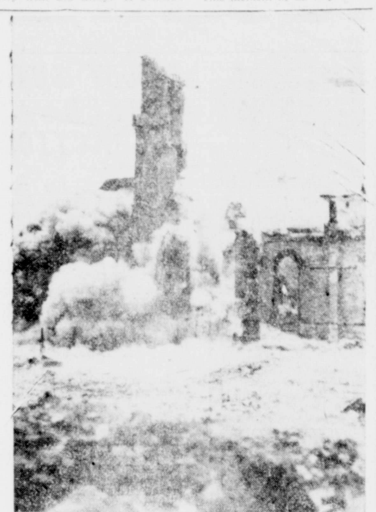
TO RISE AGAIN—American Army engineers blast a wrecked church spire in Valognes with charges of TNT. Demolition is part of engineers' assignment to tear down shell-torn buildings and clear streets of rubble to forge a path for supplies and reinforcements. (U. S. Signal Corps Photo).
