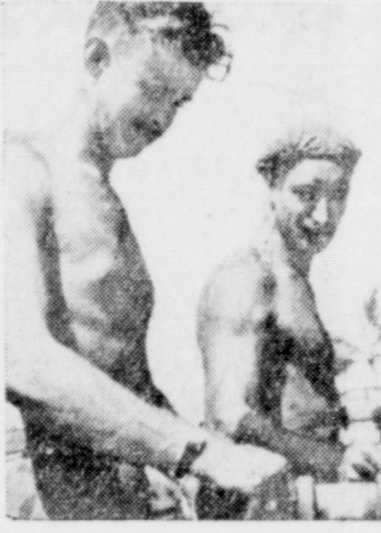
GOOD AT HOME—If and when these Seabees get home after the war, they'll be good around the house. All shipfitters, they're assembling plumbing for a hospital unit in the South Pacific. From left: Arvid Nelson, Baldwin, L. I.; Henry Dosey, Chicago, and Glenn Rankin, Hot Springs, Ark.
