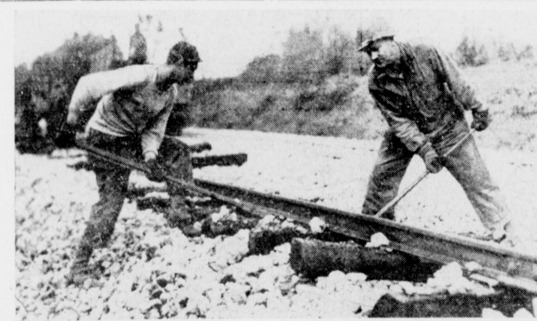
WORKING ON THE RAILROAD—Raising the rails of a wrecked roadbed in Southern Italy, Pvt. George Biegle of Evansville, Ind., and Pvt. George Roberts of San Bernardino, Cal., rapidly restore the line to help expedite flow of material to new fighting front.
