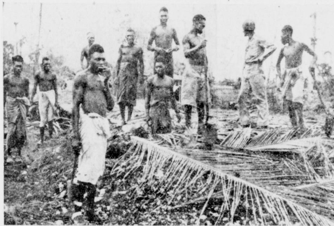
TIME OUT—Natives of New Guinea who are accustomed to working in the hot, humid climate construct a converted bomb shelter in rapid time under the direction of T-3 Jesse Opperman of Detroit, Mich. Picture was snapped while the men took time out for rest and refreshment.
