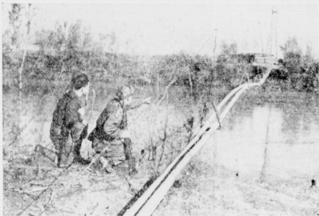
OIL FOR ITALY—Constructed and put into operation in one week, this pipeline conducts oil from an Italian seaport to point just behind the frontlines. High tension towers lend support and line is welded for strength and flexibility.
