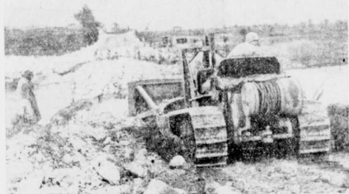
RUSH JOB—Hard-riding bulldozer helps U. S. Army engineers in Italy rebuild old Volturno river bridge wrecked by retreating Germans. Temporary ponton bridges handle river traffic, but there is danger that they may be washed away.
