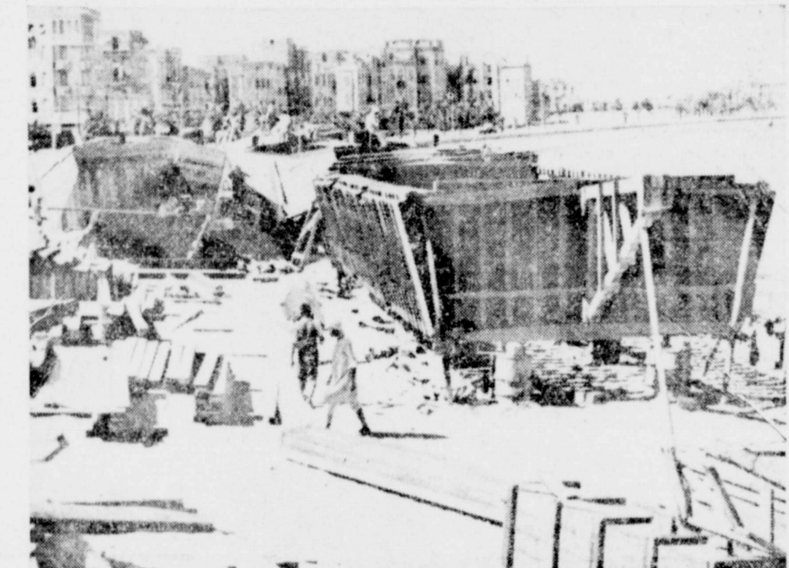
BARGES TO CARRY 200 TONS - With materials sent from America, local labor is used at Alexandria, Egypt, to build new type of naval lighter. Constructed of wood and canvas, flat-bottomed barges can carry 200 tons of cargo.
