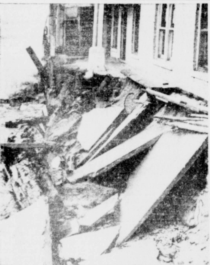
LAKE GETS FRISKY —First of the winter's gales lashed over Lake Michigan and whipped up highest lake level in years. High waves smashed retaining wall and sidewalk on Chicago's north side and threatened apartment house foundations.
