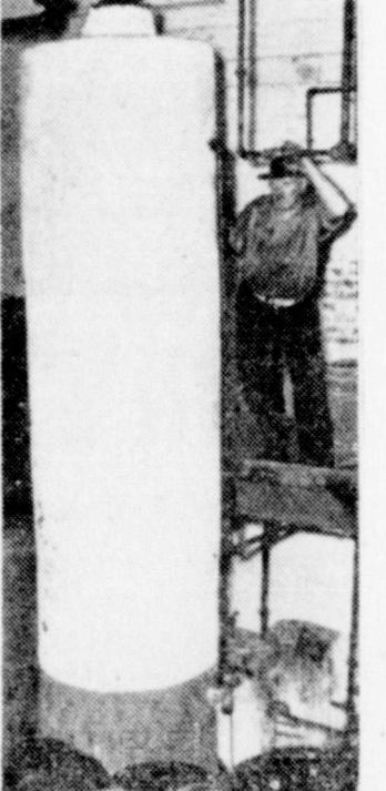
DEODORIZING TANK IS AN AID IN REFINING.
