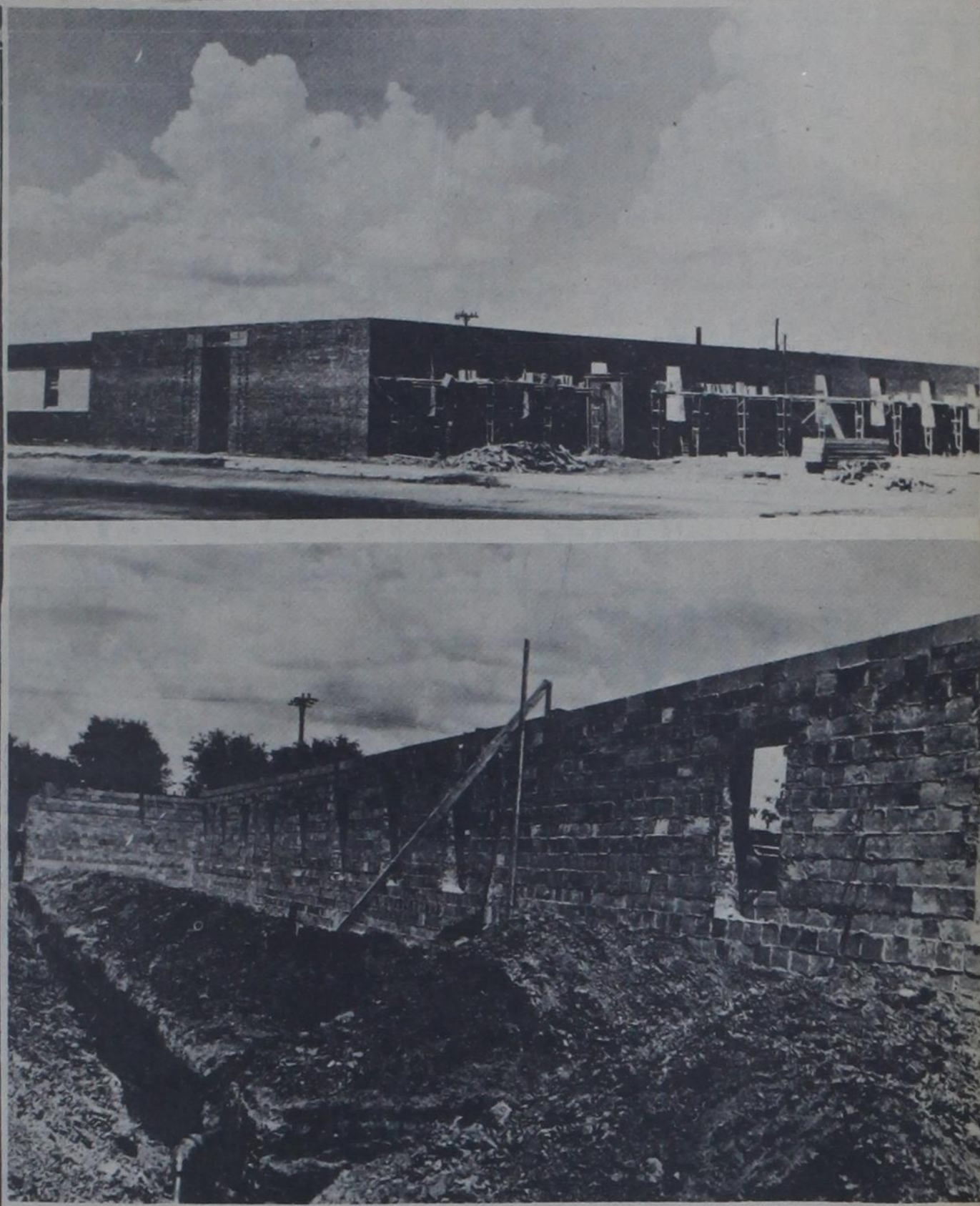
'WING' TAKES SHAPE — Construction progress has seemed rapid on the new 16-bed wing of Plains Memorial Hospital, with the exterior walls already up. Inside the walls, the wing's complex plumbing system is being "roughed in." Lampe Construction Co. of Lubbock started the $222,000 project last month, and has 10 more months to complete it.
