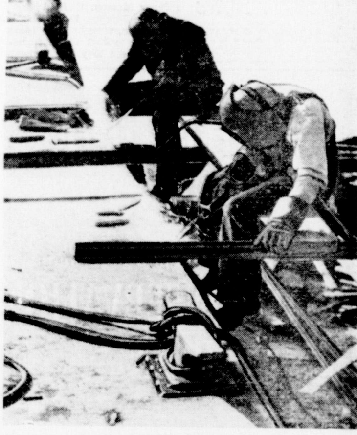
HOODED KNIGHTS OF FLAME —Welders put the finishing touches to an oil barge as they weld deck plates in place.
