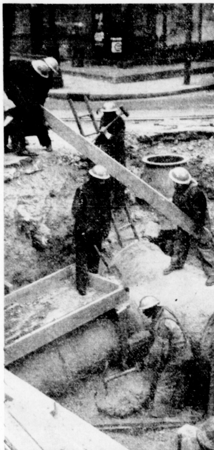
AIR RAID REPAIRS--A New York corps of trained technicians is practicing making emergency repairs--as on water main above--in case enemy air raiders ever attack the city.
