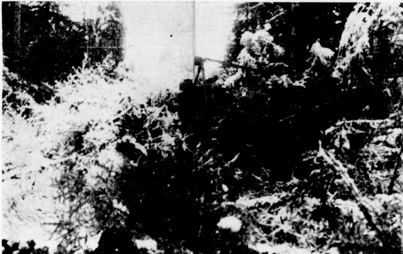
BUILD ALASKAN ROADS—Through this twisted mass of snow covered trees and branches the U. S. Army tractor sticks its nose as engineers undertake the herculean task of road building for defense in Alaskan interior.
