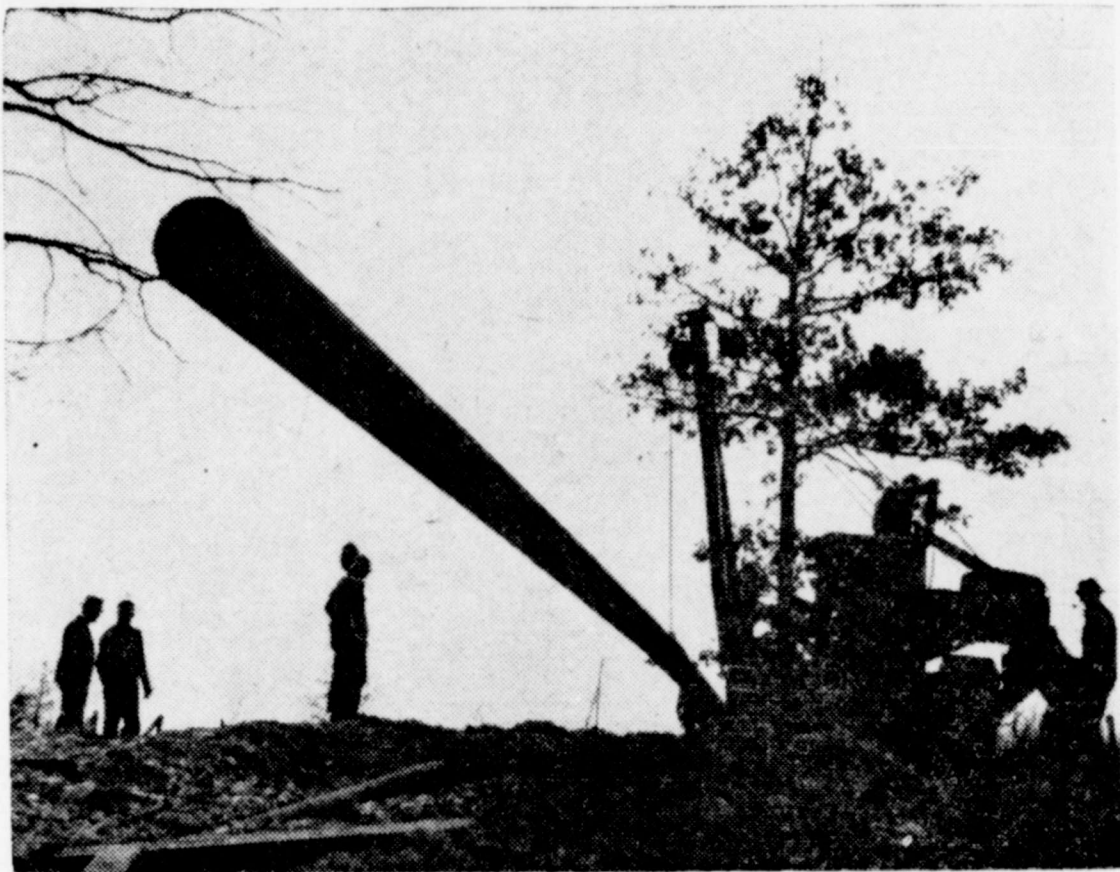
This isn't a "Big Bertha" or any other variety of seige gun, it's an old pipe being lifted to a new position. Construction of the Grand River dam north eastern Oklahoma, near Vinita, caused the relocation.
