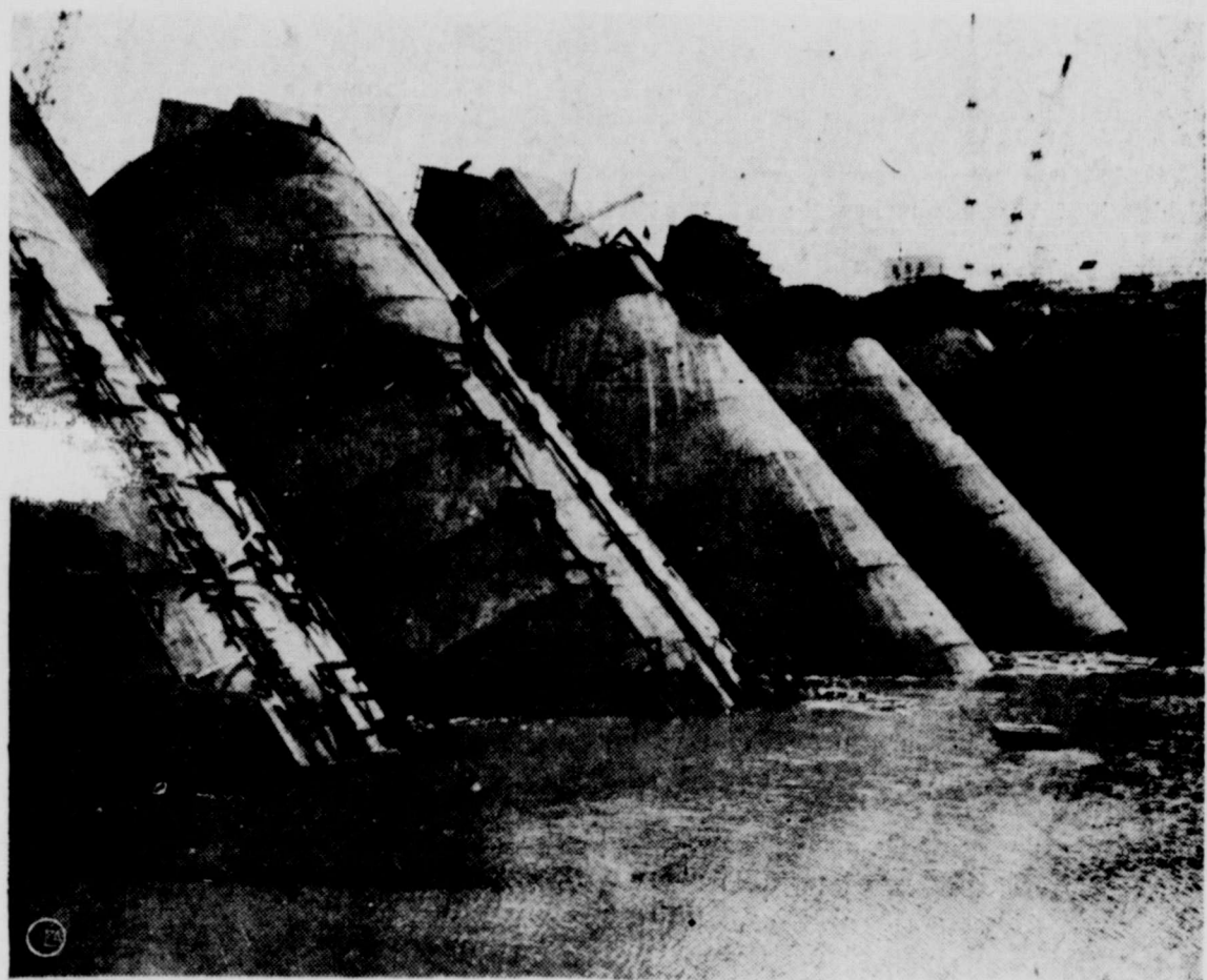
With the last gate just closed at the Grand River Dam, water begins rising forming a lake which will eventually bury three roads and two bridges. Workmen closed the 6,000-foot long, 150-foot high dam protected from the Oklahoma national guard by a federal injunction. NEA Telephoto.
