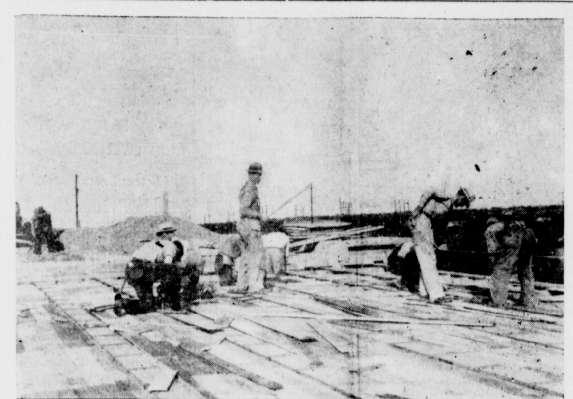
Workmen here are shown building forms for the flooring of the new overpass at Eighth street and Katy railroad, which is nearing completion by the Jensen Construction company. The structure, one of the most beautiful in the state, will be opened about June 1. It carries the new route of Highway 80, the Bankhead, over the Katy tracks where once a small wooden bridge spanned the tracks.
