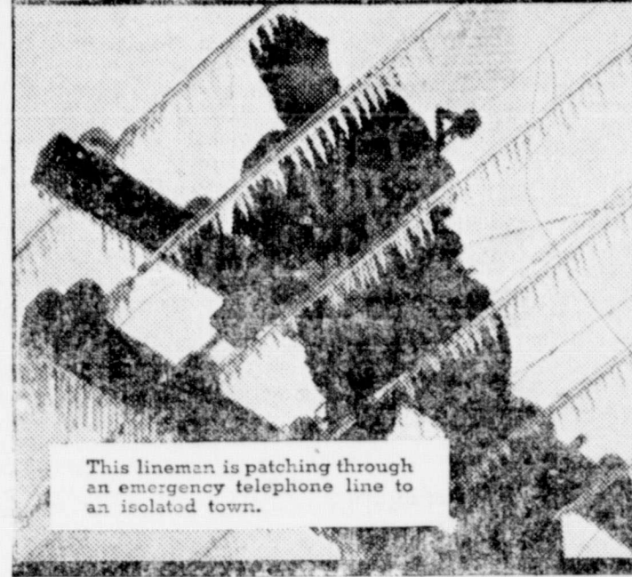
Repair crews, rushed into January sleet storm area, found miles of telephone line flattened by ice.
