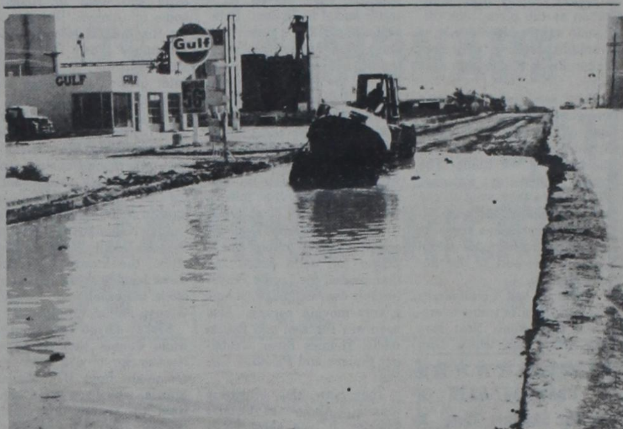
LAKE BEDFORD — Highway construction workers were plagued with more woes Saturday morning when this water truck dropped into a hole on East Bedford, re-breaking a water main and turning a section of the street into a lake. Ned Smith, city director of public works, said the two-inch main already had been ruptured once, and that the city had repaired it Friday afternoon
