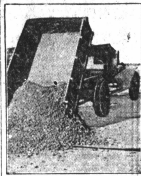
One Type of Road—Truck-Load of Hot Concrete Being Dumped Ready for Surfacing.
