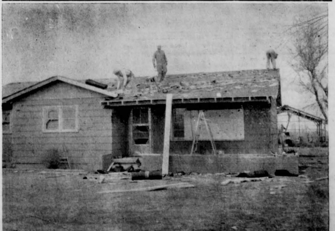
REPAIR WORK STARTS —Four days after the tornado at Sunnyside carpenters began repairing the home of Mr. and Mrs. Weldon Bradley (above). Their next door neighbor, Mrs. Howard Bridges was planning Saturday on starting soon rebuilding their seriously damaged home. Her husband is still in Castro County Hospital recovering from tornado injuries.
