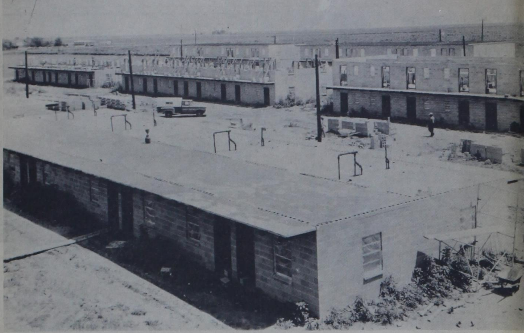
A SMALL CITY is taking shape at the site of the Castro County Migrant Housing Project, the biggest project of its type in the US. Construction has reached the second story level on many of the apartment buildings. The Castro County Agricultural Housing Association, Inc., and H. A. Padgett Construction Co. of Lubbock, contractor,
