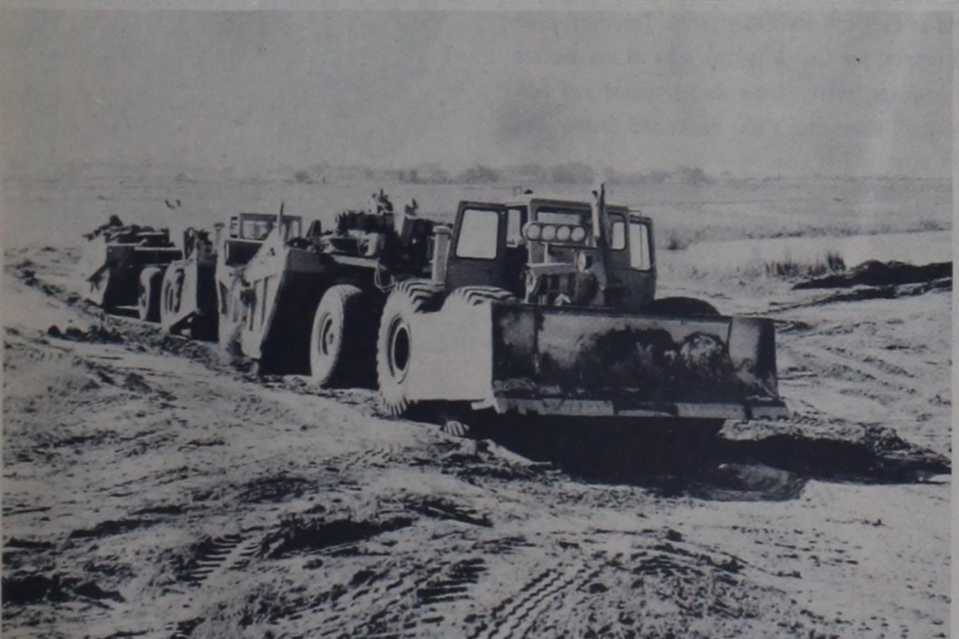
EARTH-MOVING FINALLY IS IN FULL SWING AT RECREATION CENTER . . . Two power-wagons aid each other in carving future golf course
