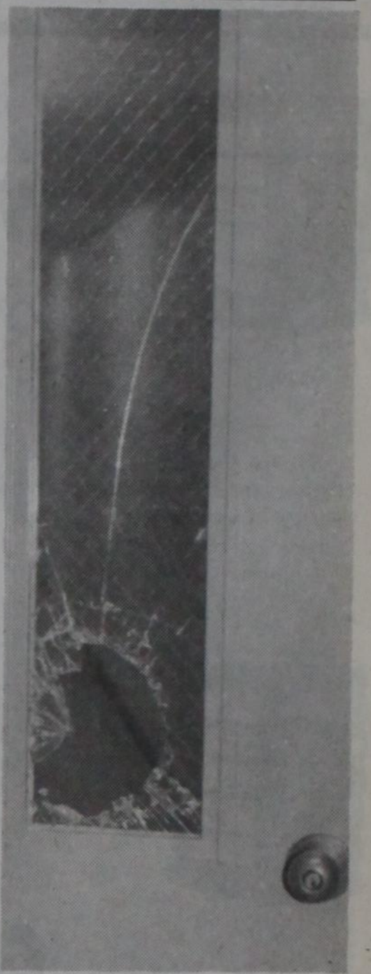
ACCESS DOOR to the underground tunnel was the source of trouble for burglars trying to get back out of the bank in a break-in early Monday at the First State Bank of Dimmitt.
