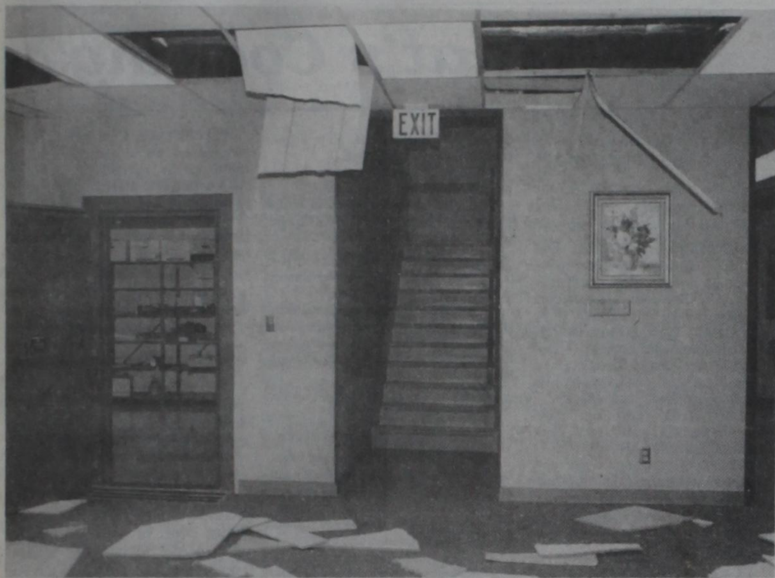
CEILING TILES aren't where one would usually expect damage in a bank burglary, but apparently the intruders in Dimmitt's First State Bank over the weekend were either trying to get into a vault,
