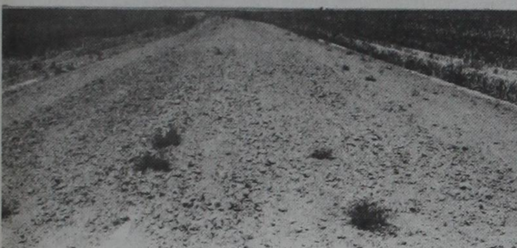
This past year, through the GPCP program, the District assisted a local landowner in the layout and construction of two diversion terraces. These diversions were installed to help control concentration of outside water that was cutting washes and gullies across the producers fields. Other practices that are cost shared under the GPCP program include pasture planting, range seeding, parallel terraces, waterways, windbreak trees and critical area shaping. Also this year 100 acres were seeded and established to permanent pasture under the GPCP program. Anyone interested in a GPCP contract should contact the local SCS office in Dimmitt.
