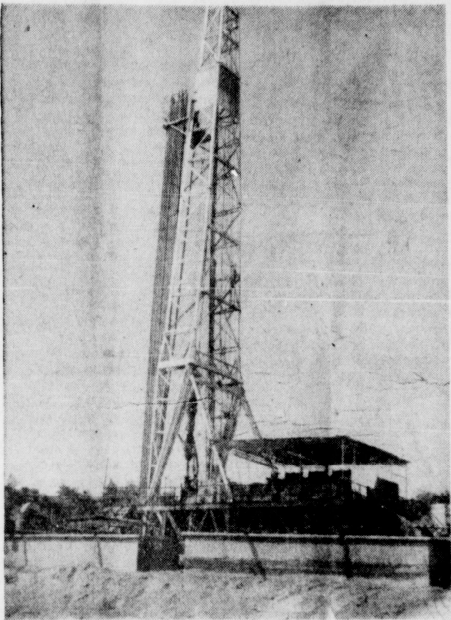
EMPIRE DRILLING COMPANY'S rotary rig No. 2 is shown on Sun Oil Co. No. 1 Menielle location, 9 miles northwest of Robert Lee. The photo was taken Monday morning when they were going back in the hole to drill deeper. Oil shows in the Menielle well are the most promising discovered in Coke County for a long time.
