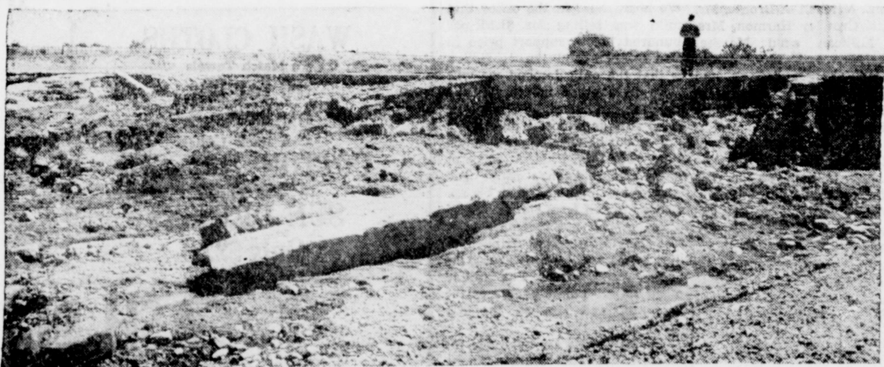
DAMAGED SPILLWAY —The Robert Lee Mountain Creek dam spillway is pictured here in its damaged condition. A flood last summer washed away considerable earth and damaged concrete stringers. Engineers and UCRA officials failed to agree on how to construct a permanent spillway until recently, when a concrete apron
