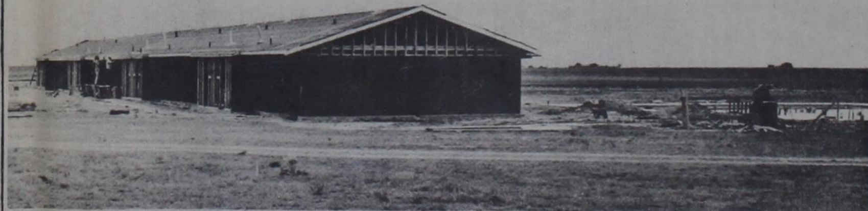
APARTMENTS GOING UP —Workers this week completed the framing and roofing of two quadruplexes in the new Ruskin Circle Apartments in Southwest Dimmitt, and are scheduled to start sheetrocking the individual rooms next week. This is the first of several luxury apartment houses
