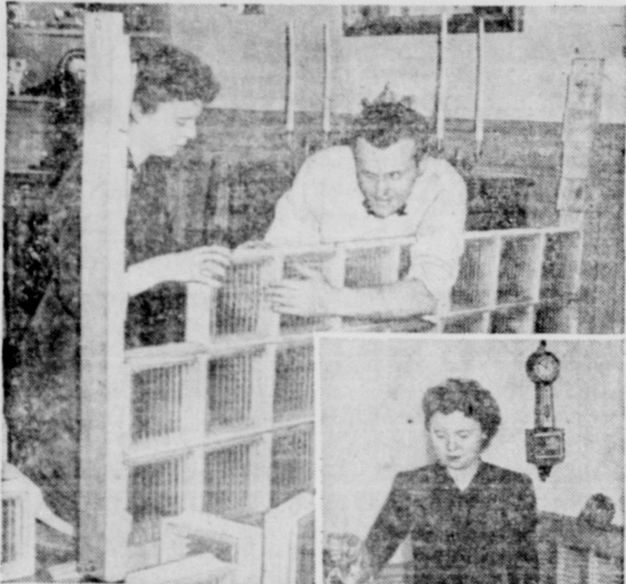
The Brothersens team up to erect a glass block and wood strip partition for the big living room of their apartment.
