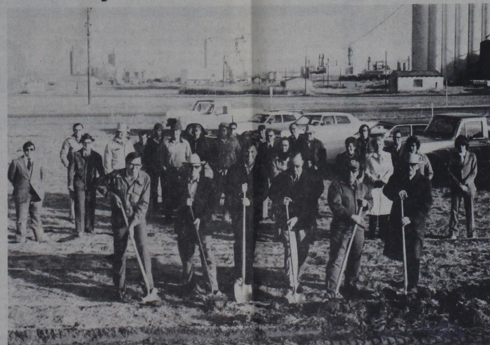
GROUND-BREAKING CEREMONIES for Hays Implement Co. were conducted Monday morning at the eight-acre building site on US 385 South. Manning shovels are [from left] owners Doug, Jim and David Hays, Parts Manager Boyce Carter, Service Manager Randy Hunter, and Mayor Elmer Youts. In background are company employees, spouses, and Chamber of Commerce and city officials. The new 8,700 sq. ft. building, hoped to be completed in June, will be almost four times as large as the present Hays Implement Co. building.
