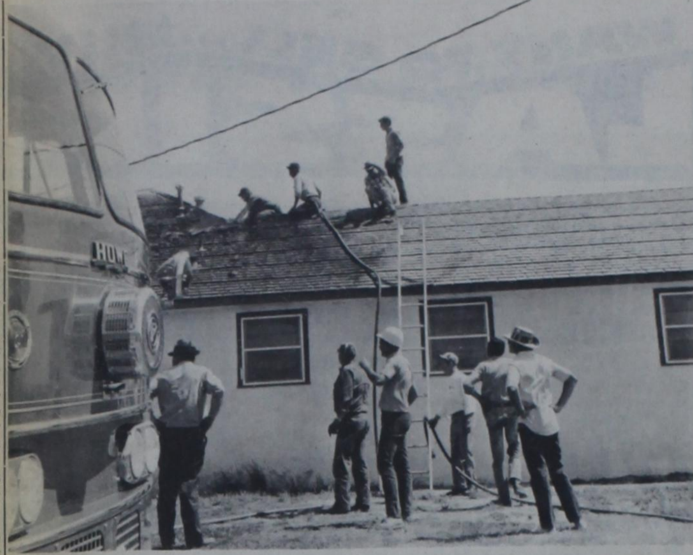
ROOF-BLAZE —The James Burnam home near the "Y" intersection of US 385 and State 194 received flame and smoke damage when the roof caught fire last Wednesday afternoon. Here, Dimmitt volunteer firemen peel shingles from the roof as they trace the path of smoldering cinders. Although the cause of the fire has not been
