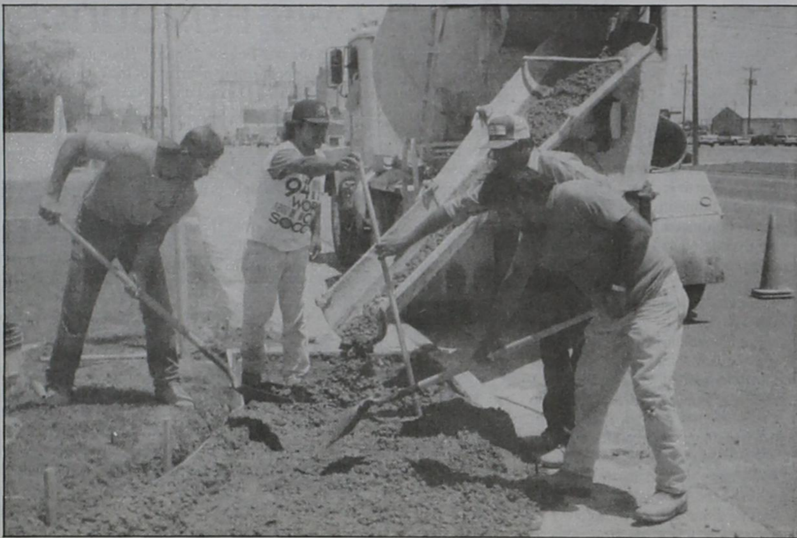
ACCESSIBLE SIDEWALKS —Workers for Concrete Constructors of Plainview work on a handicap-accessible sidewalk Friday at the corner of NW Fourth and Bedford in Dimmitt. The sidewalk, with a ramp
